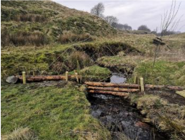
Leaky dam above Pott Shrigley
