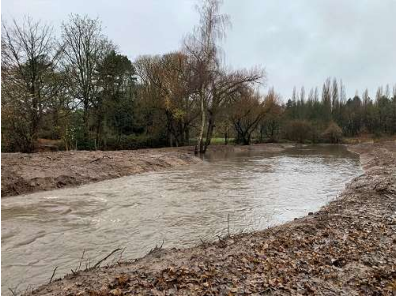
Fig. 2 Wetland created alongside the River Alt in Croxteth Park
